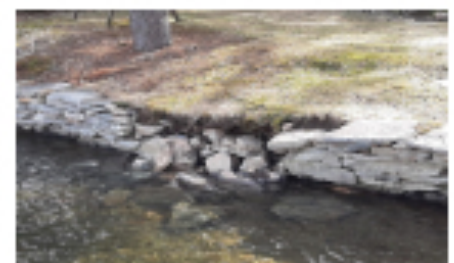
Erosion and property damage
